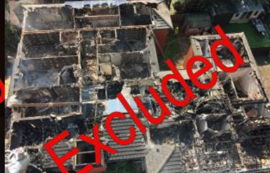
Newgrange care home 2017, Cheshunt, Herts, 2 fatalities 1 storey
